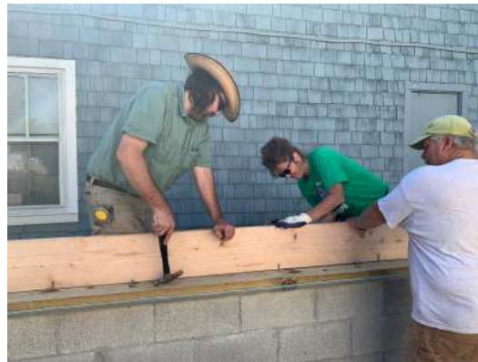
(From left to right) John Puposzar, Critical Home Repair Manager; JoAnn Hansen, Chief Executive Officer, and Jim Thomas, Construction Project Manager work on a construction site on South Locust Street.
